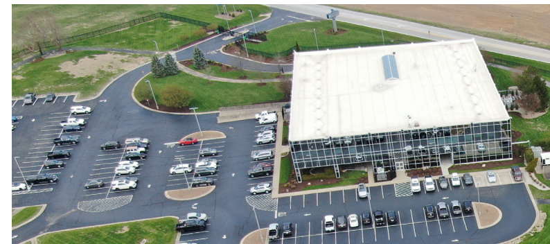
Solar array at headquarters in Owensboro, KY
